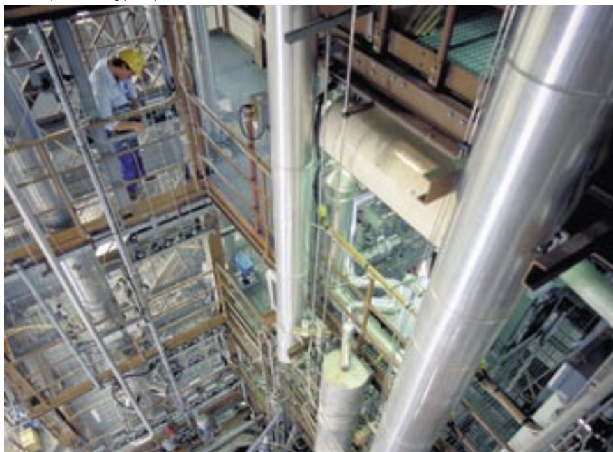
LOBI Project - Testing facility.
