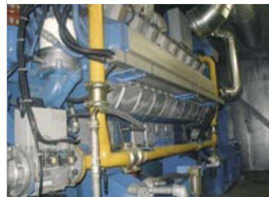
Ispra cogeneration plant.
